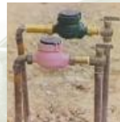
Recycled water (the purple outlet) will be used for toilet flushing and irrigation.
